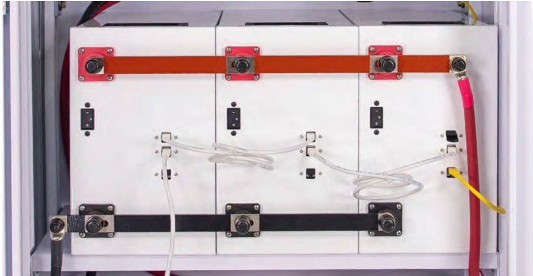
Figure 8.0 – AmpliPHI Wiring using Interconnecting Busbars
